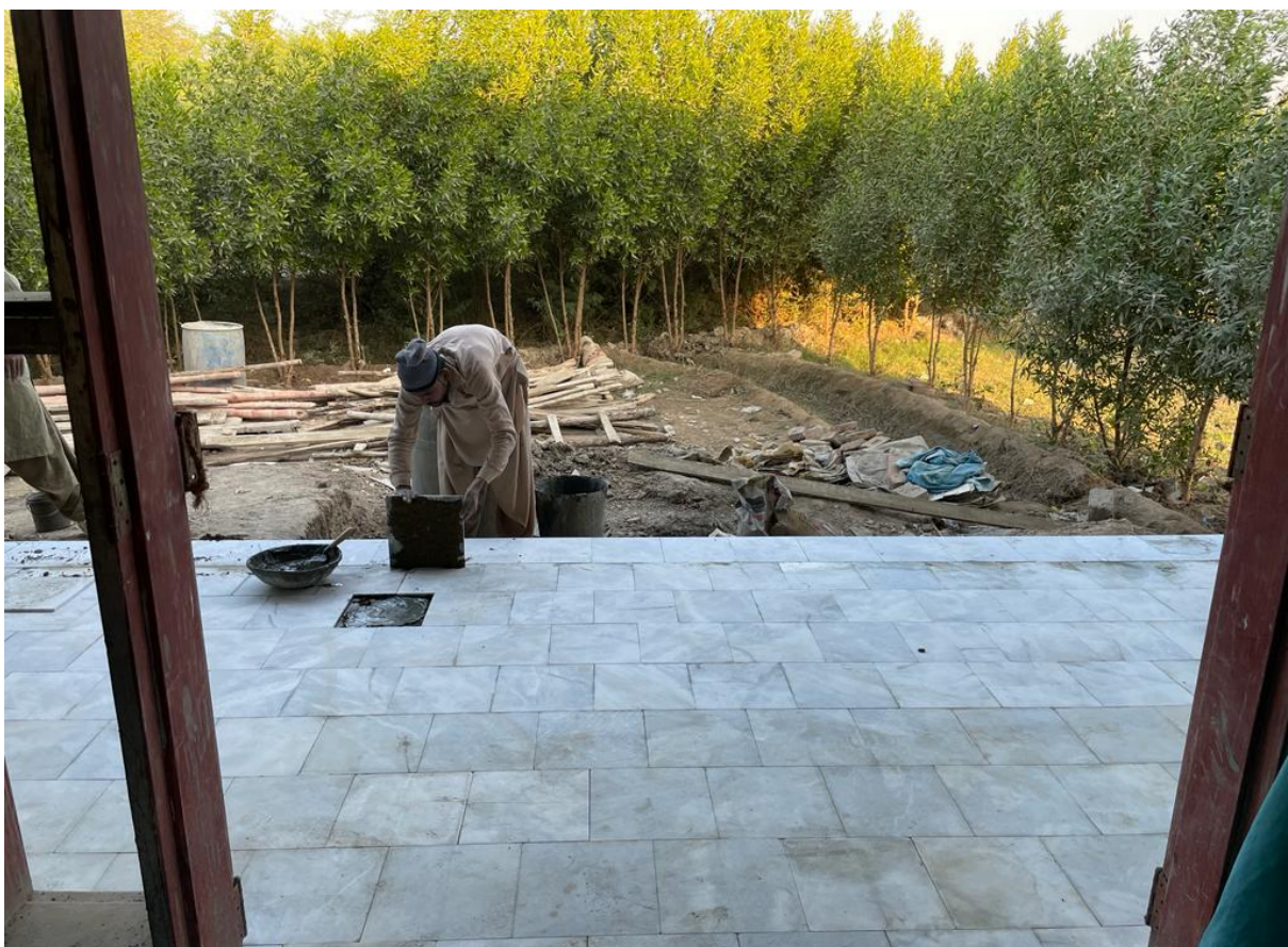
November 2022: The last tile - a construction worker adds finishing touches to the PAAS hospital verandah.
